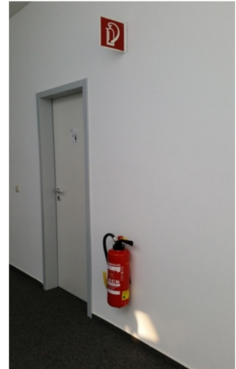
Fire extinguisher everywhere
