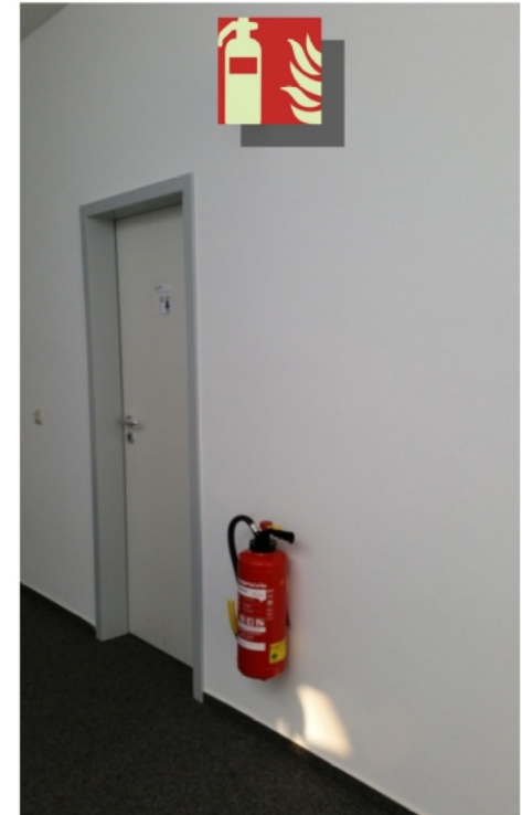
Fire extinguisher everywhere
